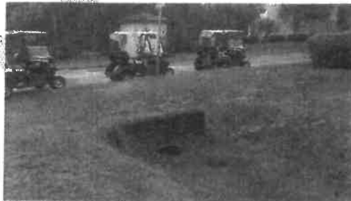
Woodlands Parkway at Cypress Estates 1-clear mouth of culvert $ 685.00
