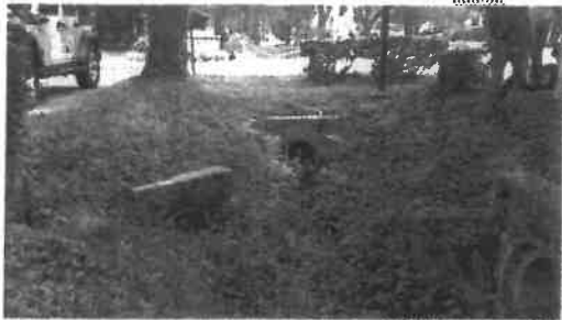
East Lake Woodlands Parkway at Town Center-clear ditch $ 1,245.00
