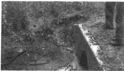
Course access rd between 4 and 15 N.-repair erosion $ 1,860.00
