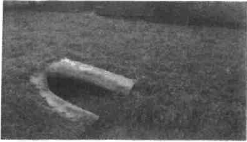
Woodlands Parkway at Cypress Estates 1-clear mouth of culvert $ 550.00
