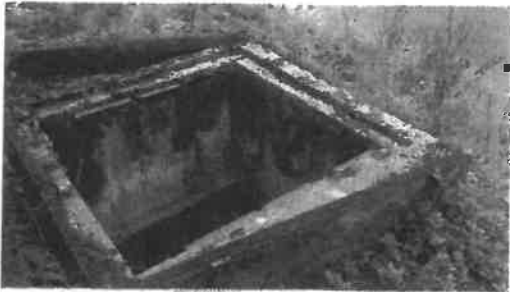
Nursery Rd-fabricate grate for wet well.. Proposal requested by East Lake Water.
